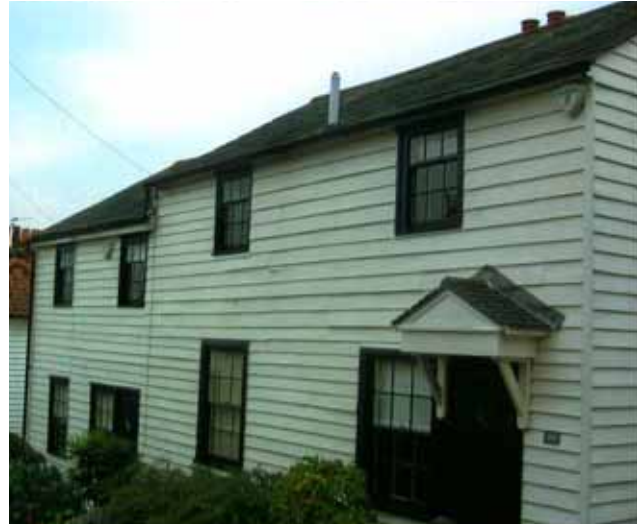
This fine example of traditional building materials is to be found at 20 Kings Hill with traditional slate roof, wooden weatherboarding and wooden sash windows.
